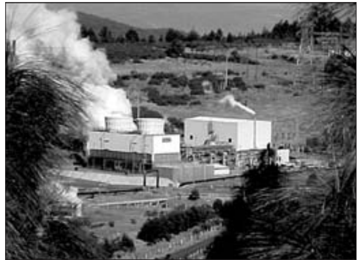
One of the four 25-MWe units of the project Los Azufres II
