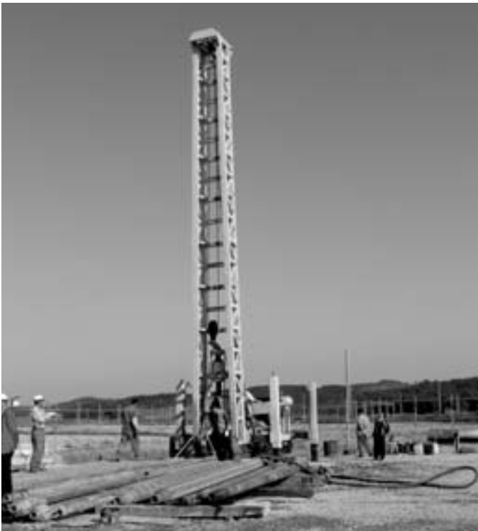
Figure 2. 2000 m deep production well in the Pohang project site, Korea (28 October 2004)
